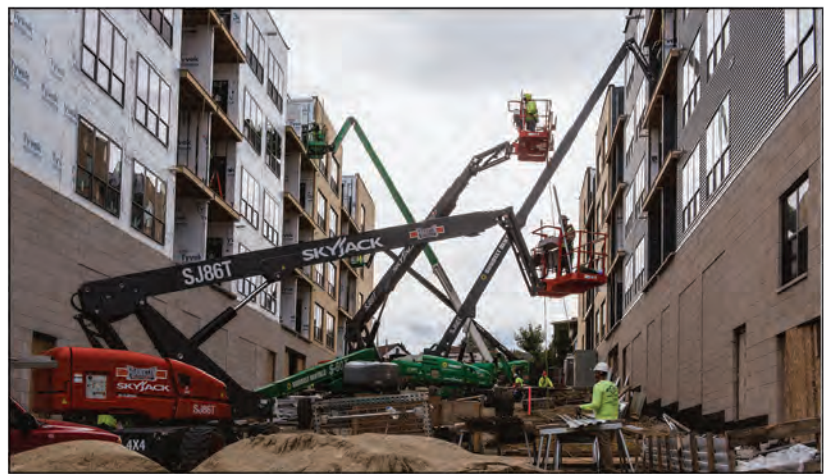
Construction crews working on the exterior brick, siding and windows. The first phase of this project is expected to be complete in December.
