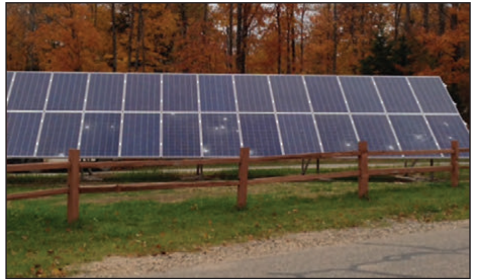
This photo shows the vandalism on the solar panels located at the AODA building.
